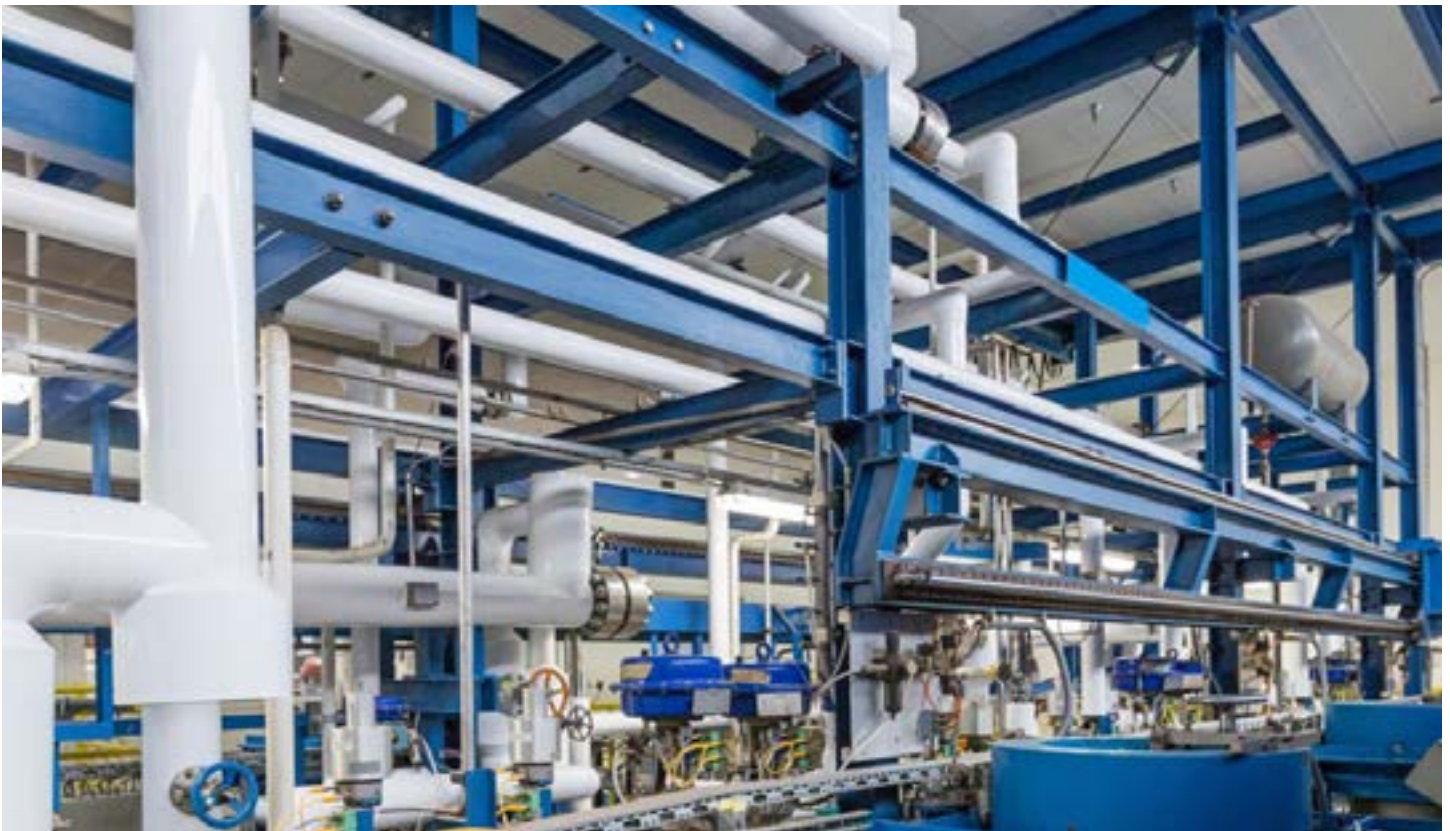
Valensa's supercritical carbon dioxide extraction facility, Eustis, Florida
